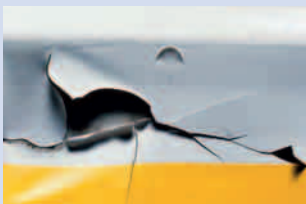
Film shrinkage and tearing
