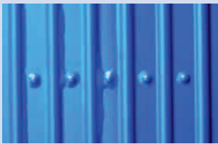
Lifting around rivets and bridging of corrugations
